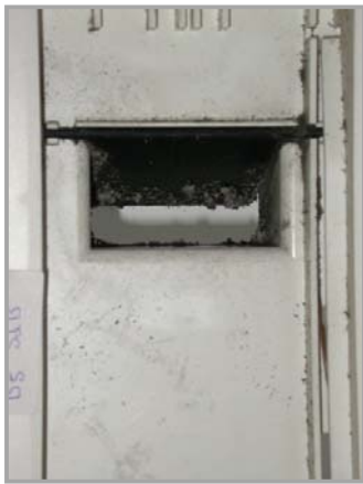
Figure 18: Fixed (not humidity-controlled) exhaust unit
