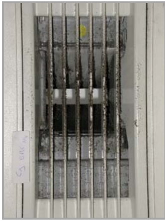
Figure 8: Kitchen humidity-controlled exhaust unit, with protection grid
