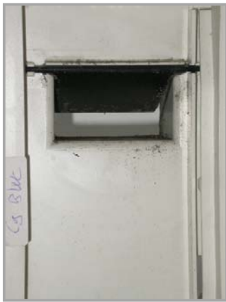
Figure 12: Fixed (not humidity-controlled) exhaust unit
