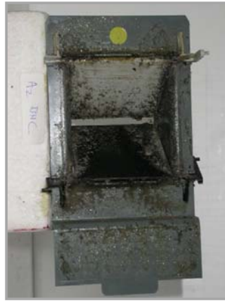
Figure 15: Kitchen humidity-controlled exhaust unit, protection grid removed
