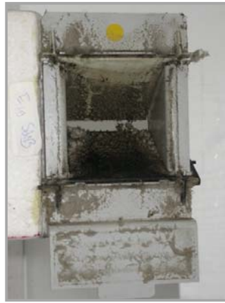
Figure 17: Bathroom humidity-controlled exhaust unit, protection grid removed
