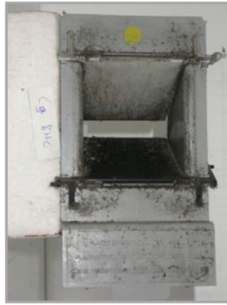
Figure 9: Kitchen humidity-controlled exhaust unit, protection grid removed
