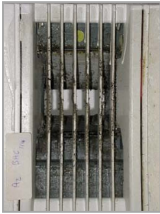
Figure 14: Kitchen humidity-controlled exhaust unit, with protection grid
