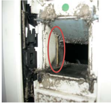
Figure 5: Shutter blocked open with a match
