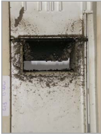
Figure 24: Fixed (not humidity-controlled) exhaust unit
