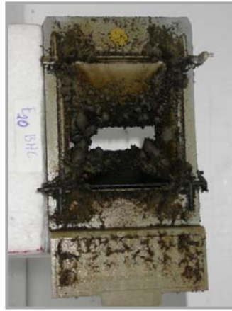
Figure 21: Kitchen humidity-controlled exhaust unit, protection grid removed
