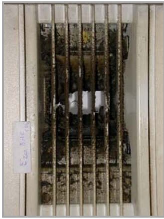
Figure 20: Kitchen humidity-controlled exhaust unit, with protection grid
