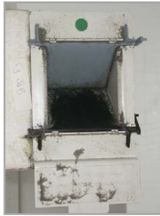
Figure 11: Bathroom humidity-controlled exhaust unit, protection grid removed
