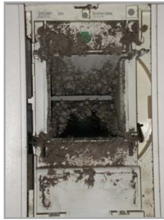
Figure 23: Hygroscopic bathroom exhaust unit, protection grid removed
