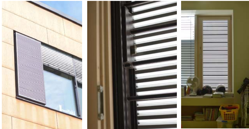
Figure 8 Window for manual night ventilation secured against rain fall and burglary but blocked by books
