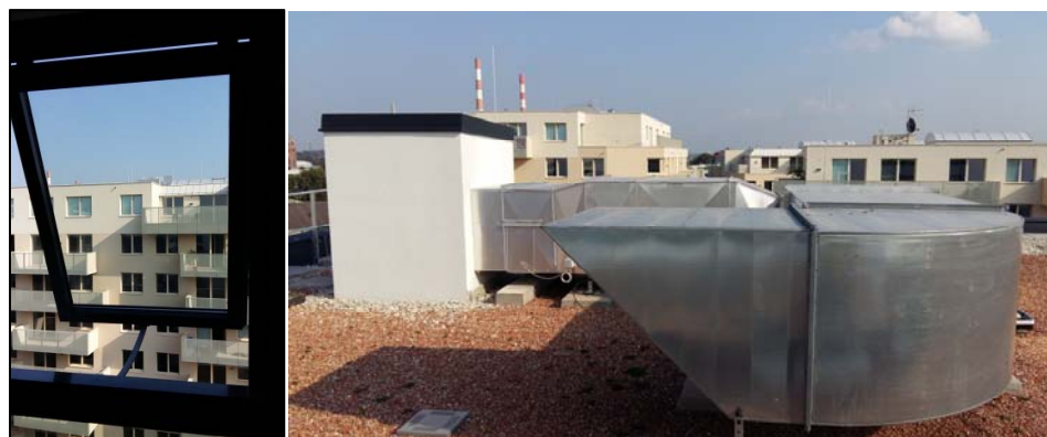
Figure 3: Air inlet window with chain actuator (left) Exhaust ventilator on roof (right)
