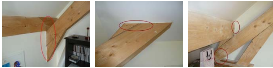
Figure 6: leakages at the junctions between the wood frame and the ceiling or the walls
