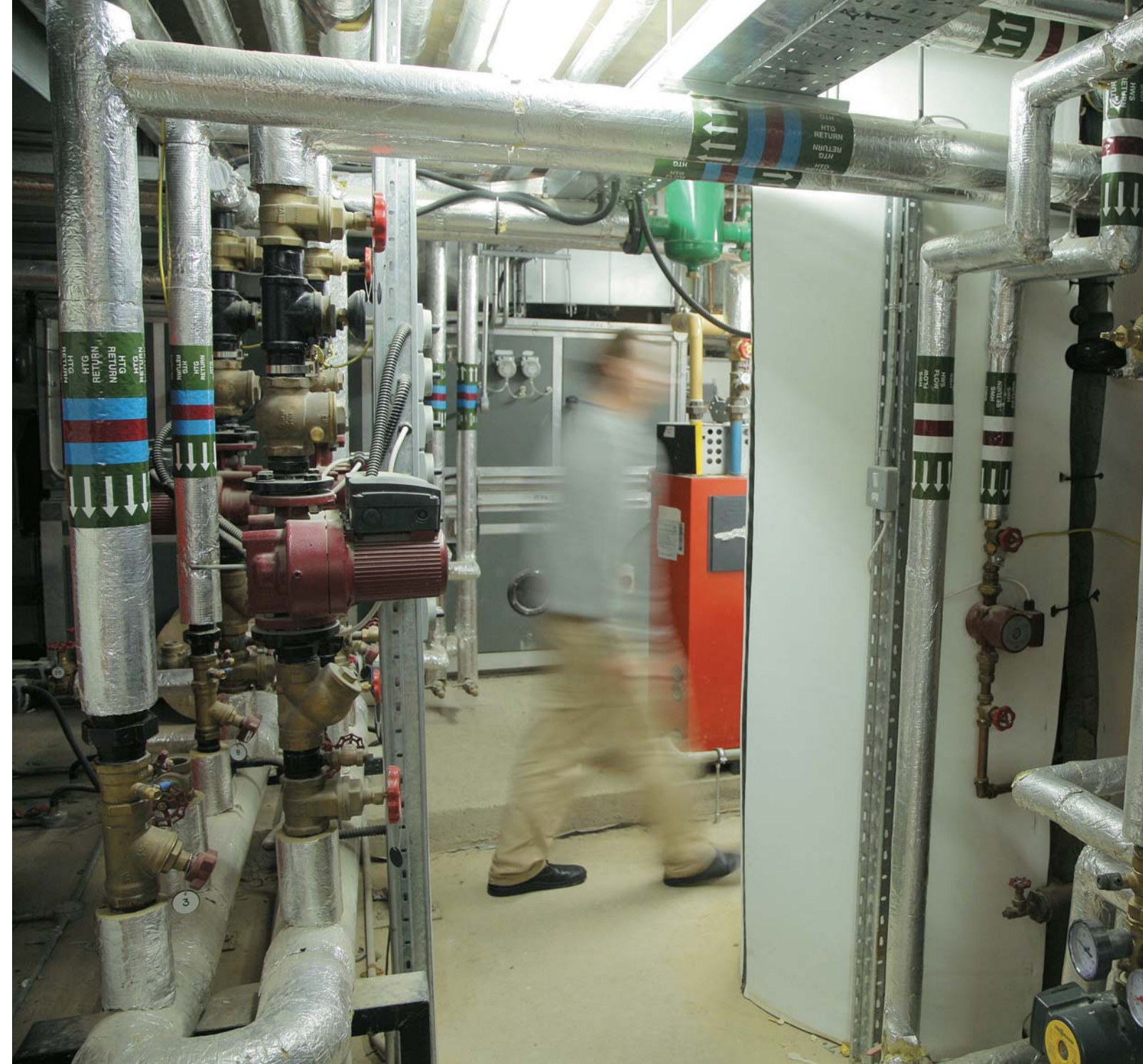
PLANT ROOM IN A NEW IRISH ENERGY EFFICIENT DEVELOPMENT CONTAINING A GROUND SOURCE HEAT PUMP, GREENWATER STORAGE TANK AND BUILDING MANAGEMENT SYSTEM.
