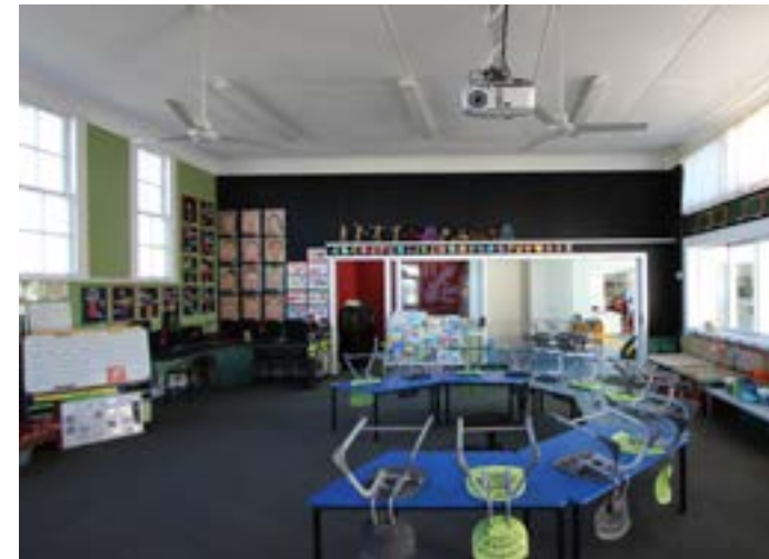
Cross ventilation and ceiling mounted fans
