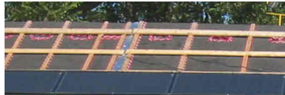
Figure 1. Photo of the BIPV-T installation found at the Northern Light Canadian Solar Decathlon 2005 house.
