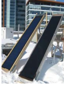
Figure 14. Left: experimental BIPV/T setup right: solar air collector.
