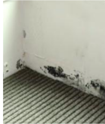
Figure 26: Mold growth on interior wall and damaged carpet due to air and water leakage (O'Brien & Artigas, 2024)
