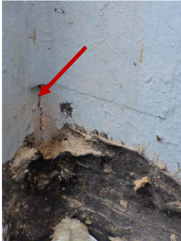
Figure 25: Breach in fluid-applied air barrier (O'Brien & Artigas, 2024)
