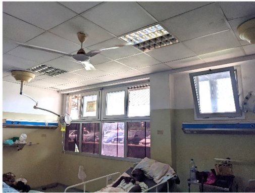
(a) Ventilation openings in the TH Emergency ward. Sliding windows and bottom-hung casement windows.
