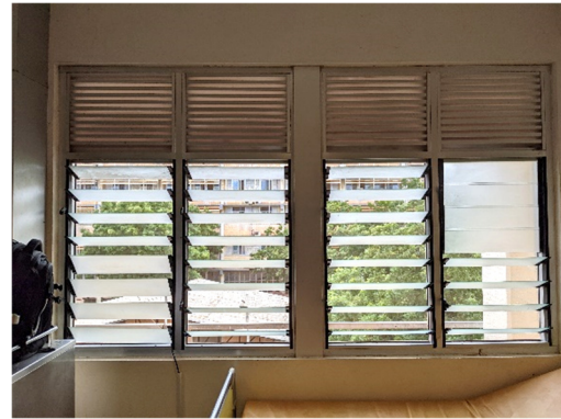
(b) Ventilation openings in the TH Post-natal ward. Adjustable glass louvre blades in lower portion with open fixed metal louvres in upper portion.
