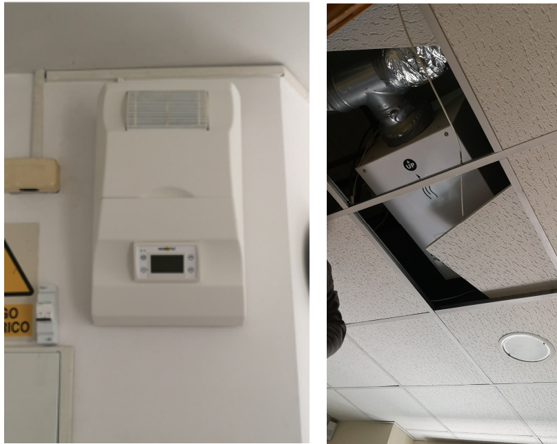
Figure 4: a) Model CTA1502365 installed in buildings A and C; b) Equipment 500 V1 installed in Building B.
