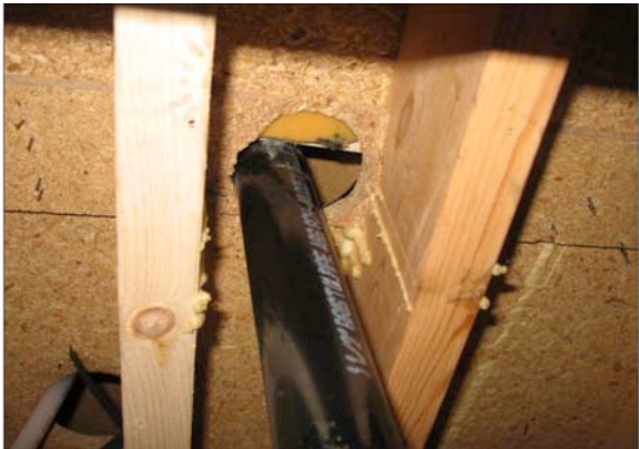
Drain line in floor (from below), leakage associated with large hole in floor relative to pipe diameter
