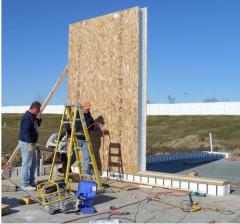
Figure 4 Placement of the first SIPs wall panel on the foundation wall sill plate.
