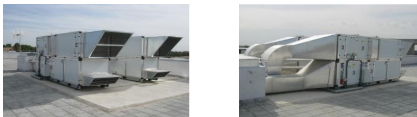
Fig. 4. Mechanical Ventilation system in an Andalusian school. Roof tops
