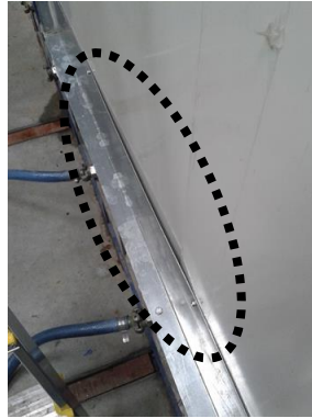
Figure 7: Wall panel deformation due to the pressure difference in depressurization test
