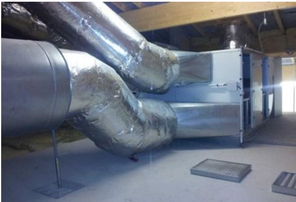
Figure 3 : The air handling unit of the ventilation system
