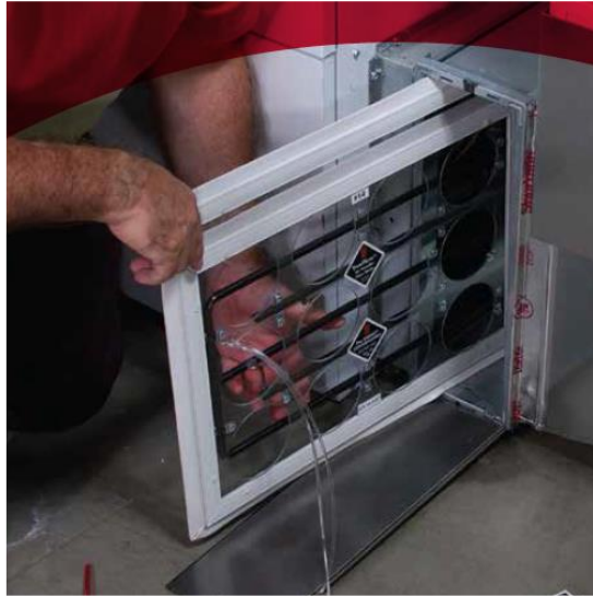
Fig. 3. Air handler flowmeter temporarily mounted in the place of air filter (The Energy Conservatory, 2014)
