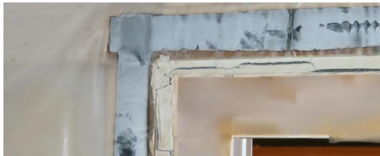
Figure 6. Joint sealant around a window.
