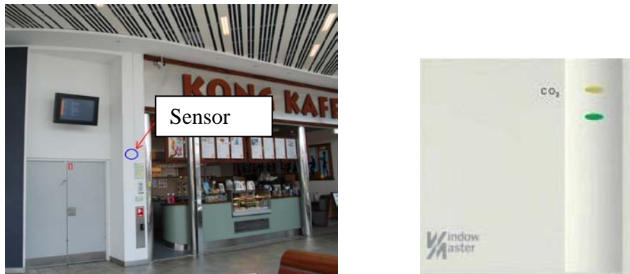
Figure 8. Example of placement of temperature/CO2 sensor and detail showing the sensor.
