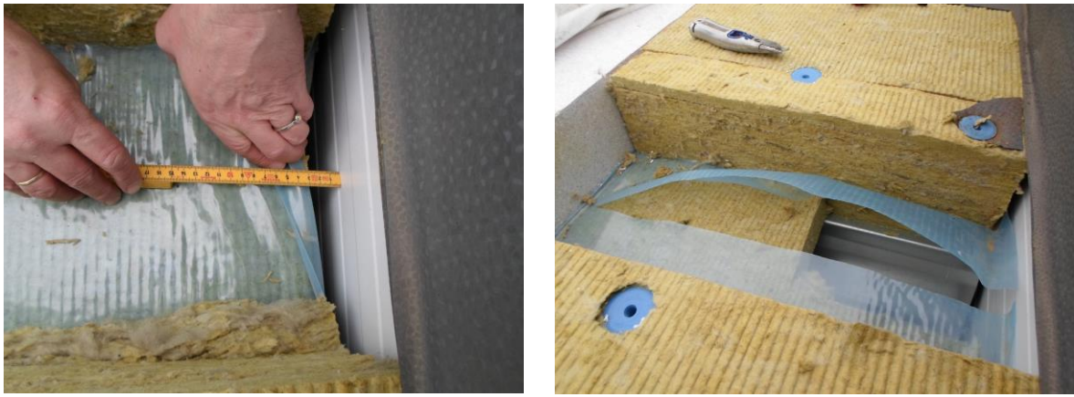
Figure 5. Lacking airtightness of the joint between the vapour barrier of a compact roof and the sandwich wall-element of a large building. Bloating vapour barrier caused by internal overpressure given in the picture to the right (Pictures: T. Bøhlerengen).
