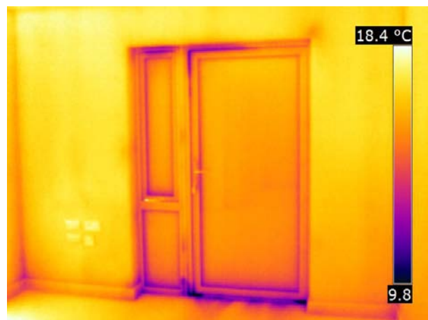
(b) Thermal image of balcony doors corresponding to photograph (a)
