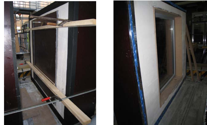
Figure 2a. calibration setup for measuring extraneous air leakage of the setup. Figure 2b. Installation of aluminum window frame and wood reveal.
