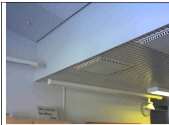
Figure 1. Ventilation duct, inlet to the library
