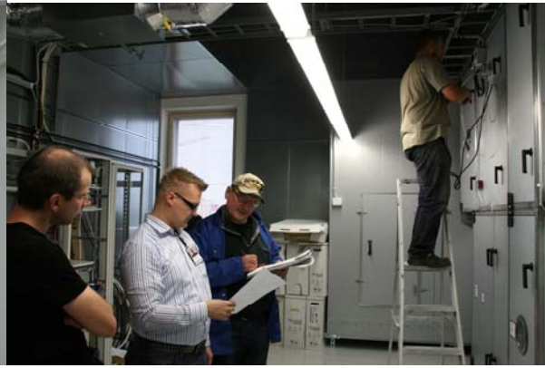
Figure 14. Measurements over the exhaust fan
