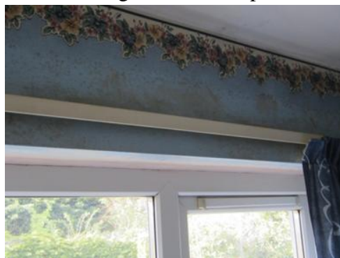
Figure 5: Staining on external wall due to condensation
