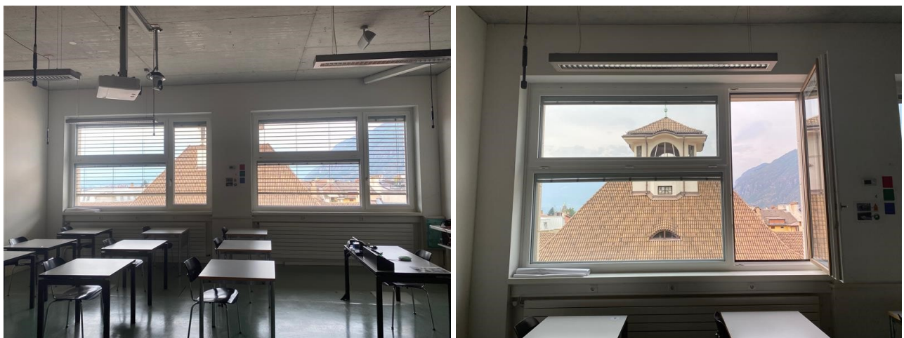
Figure 1 On the left: two set of classroom E521 windows; on the right: focus on one of the two set, with the turn window opened.
