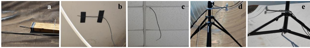
Figure 2(a-e): Monitoring system: (a) external surface temperature probe, (b) internal surface temperature probe, (c) indoor air temperature probe, (d-e) albedo in-field measurement before and after cool roof application.
