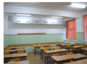
Figure 4: Inside fresh air distribution system
