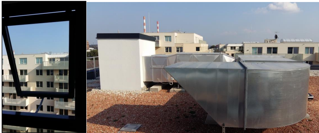
Figure 1: Air inlet window with chain actuator (left) Exhaust ventilator on roof (right)
