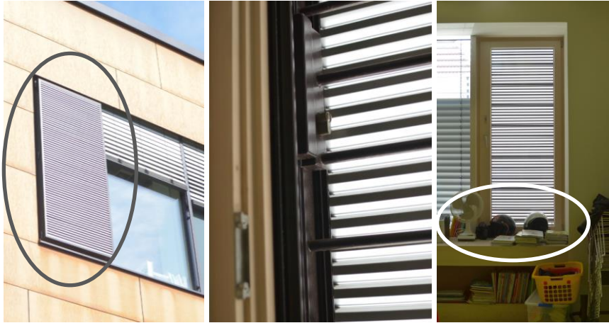
Figure 7 Window for manual night ventilation secured against rain burglary and fall but blocked by books
