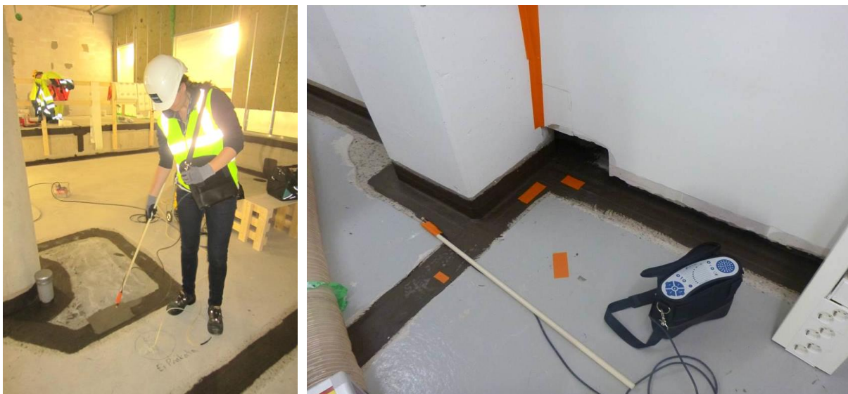
Figure 2: Air tightness renovation of concrete ground slab is done with waterproofing mass system. The tracer-gas leak test is done as part of quality control. In the picture on the right hand, in the test found leakages are marked with an orange tape, so they can be fixed.
