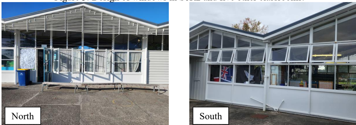
Figure 4: External door and windows for S0R2 (North) and Top-hung windows for S0R1 and S0R2 (South). Same design for five other classrooms.
