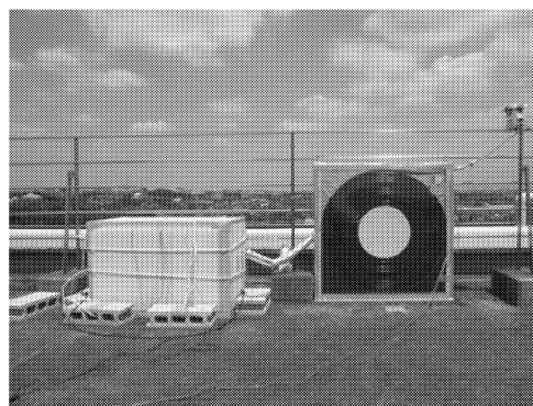
Photo 1: A simple solar water pre-heater set up
