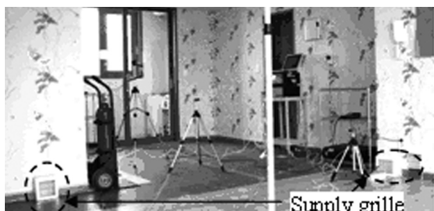
(a) Indoor air supply grille
