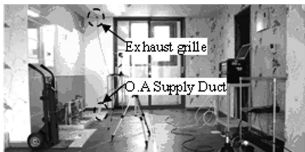
(c) Air incoming part and exhaust grille on back side
