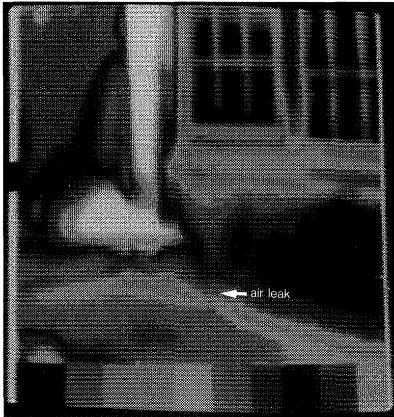
Figure 7. Window corner while pressurized.
