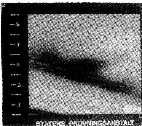
3 b) Thermogram of an area of wall/ceiling. No imposed isotherm (monochrome image).
